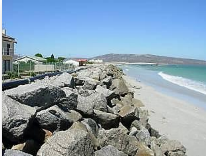
Figure 6: Example of a rock revetment protecting houses (South Africa)
