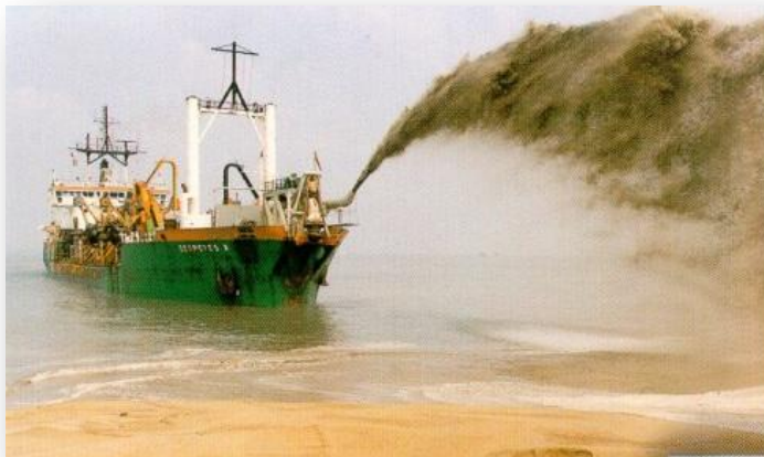
Figure.2: Beach nourishment by means of direct “rainbowing” of sand from the dredger to shore (only practical in certain areas).
