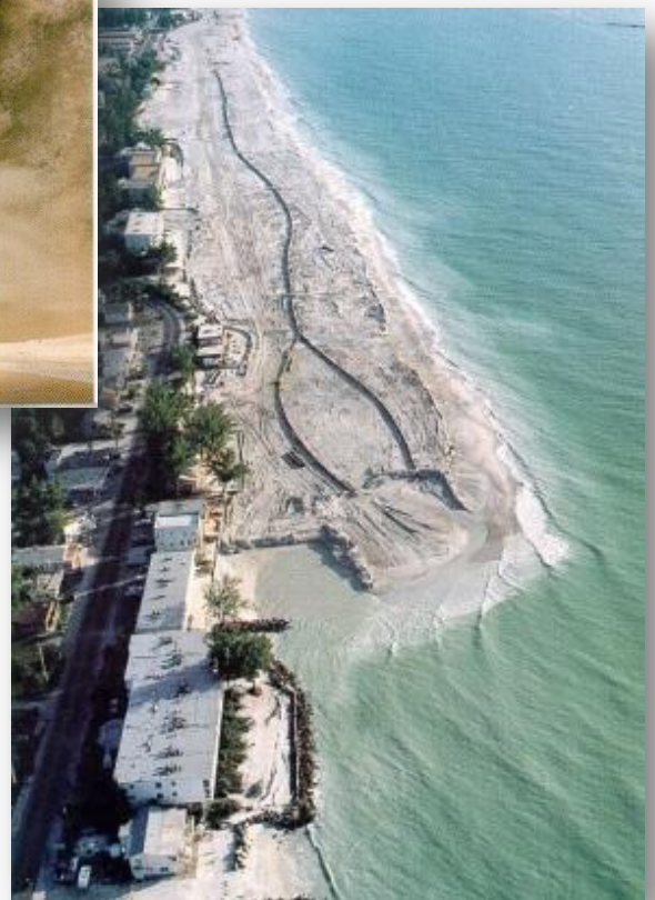
Figure 3: Beach nourishment by means of pumping sand onto the beach through a pipe system
