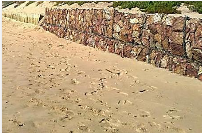
Figure 16: Example of a Gabion retaining wall structure (to protect the back-beach area)
