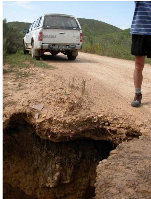
Picture 2. Soil erosion inhibiting road safety. Photo Source: Author
