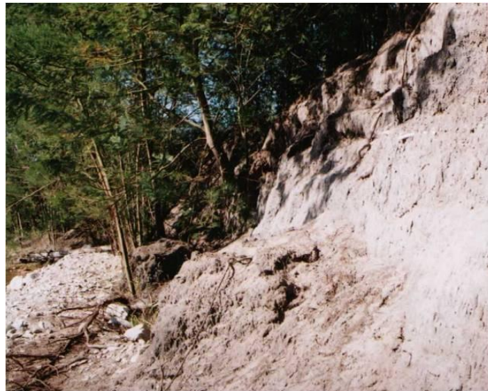
Photo 7: Bank erosion and black wattle before alien clearing in the Hudsonvale wetland (Photo by Lil Haigh) The exposed bank consists of peat
