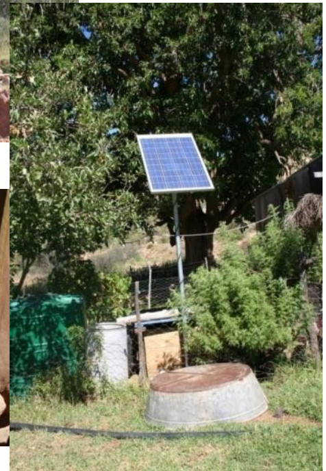
Figure 10: Solar powered water pump
